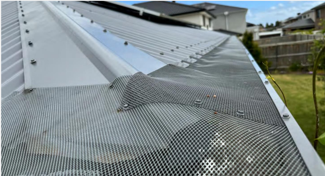
Gutter guard / bird proof mesh (Image: Water Futures)
